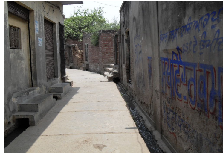
OPEN DRAINS ON BOTH SIDE OF STREET
