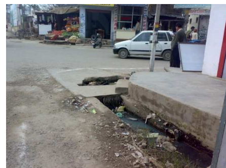
Fig no. 37: Blocked Sewerage at P.O. Chowk
