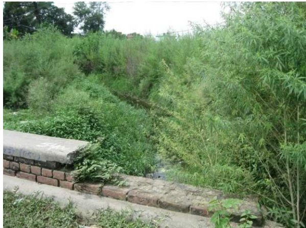
Fig No. 54:- Distributory is full of weeds, shrubs and domestic refuses instead of water supply at Jail Road
