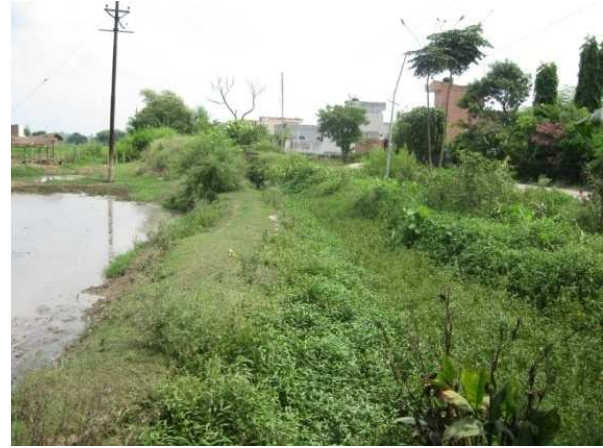
Fig No. 52:- Distributory is full of weeds, shrubs and domestic refuges instead of water supply near ITI Institute
