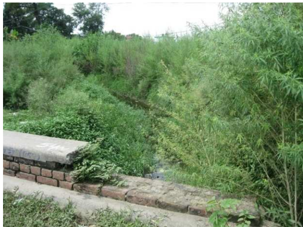
Fig No. 54:- Distributory is full of weeds, shrubsand domestic refuges instead of water supply at Jail Road
