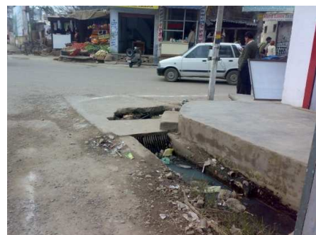
Fig no. 37: Blocked Sewerage at P.O. Chowk
